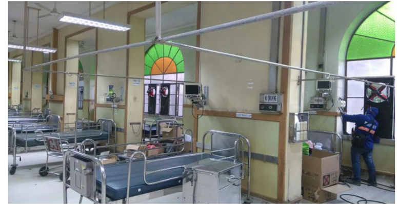
This is the PGH ward retrofitted to function as one of three Covid-19 referral centers. CONTRIBUTED PHOTO
